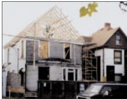
Repairing a roof can sometimes become a major job. Courtesy of CommunityWorks in West Virginia
