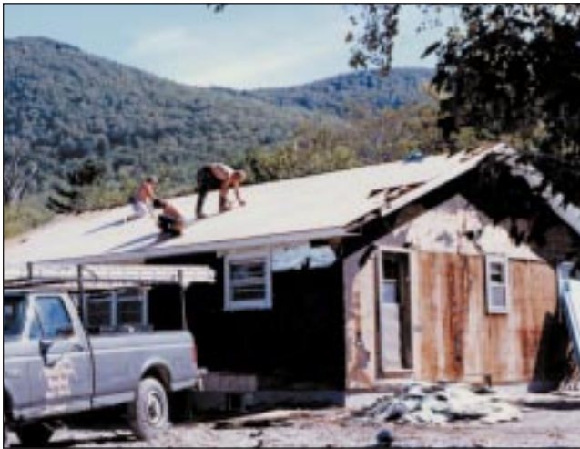
In Vermont, a crew makes progress in repairing a roof. Photo by Bert Jones
