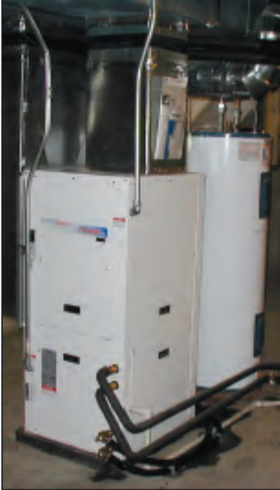
Part of a geothermal system.
